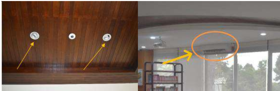
Figure 18. Use of Integrated LED Lights and AC Inverters
