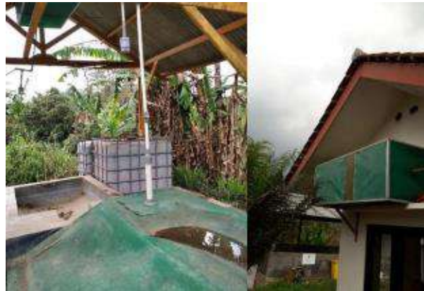
Figure 49. Biogas Installation at Universitas Padjadjaran
