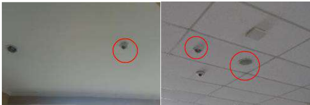
Figure 19. Integrated CCTV, Alarm, dan Loudspeaker System
