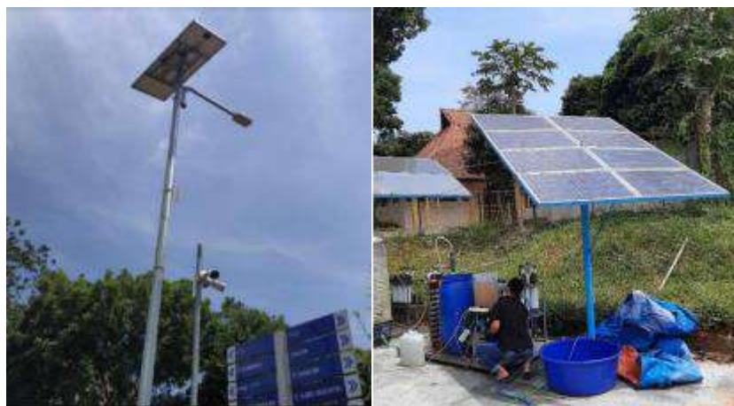
Figure 20. Use of Solar Panels for Street Lighting and Water Pumps
