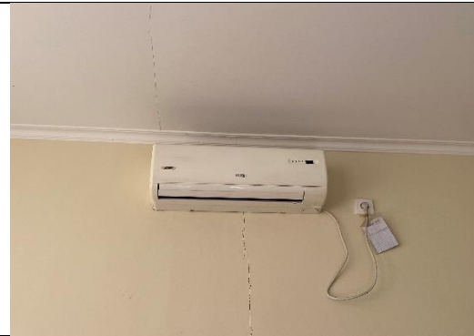
AC inverter Integrated with system
