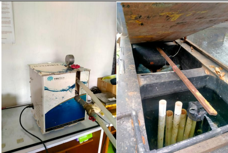
Generator and Filtration Channel of Nanobubble Technology
