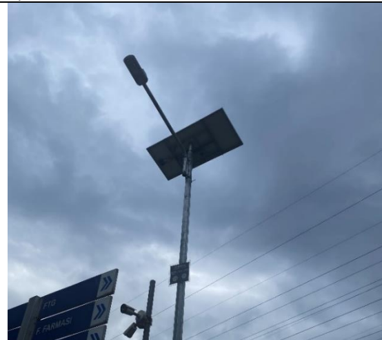
Solar panel for street lighting facilities and research
