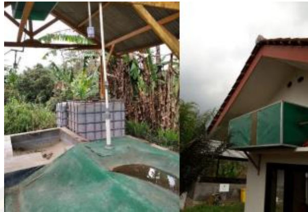
Figure 55. Universitas Padjadjaran Biogas Installation
