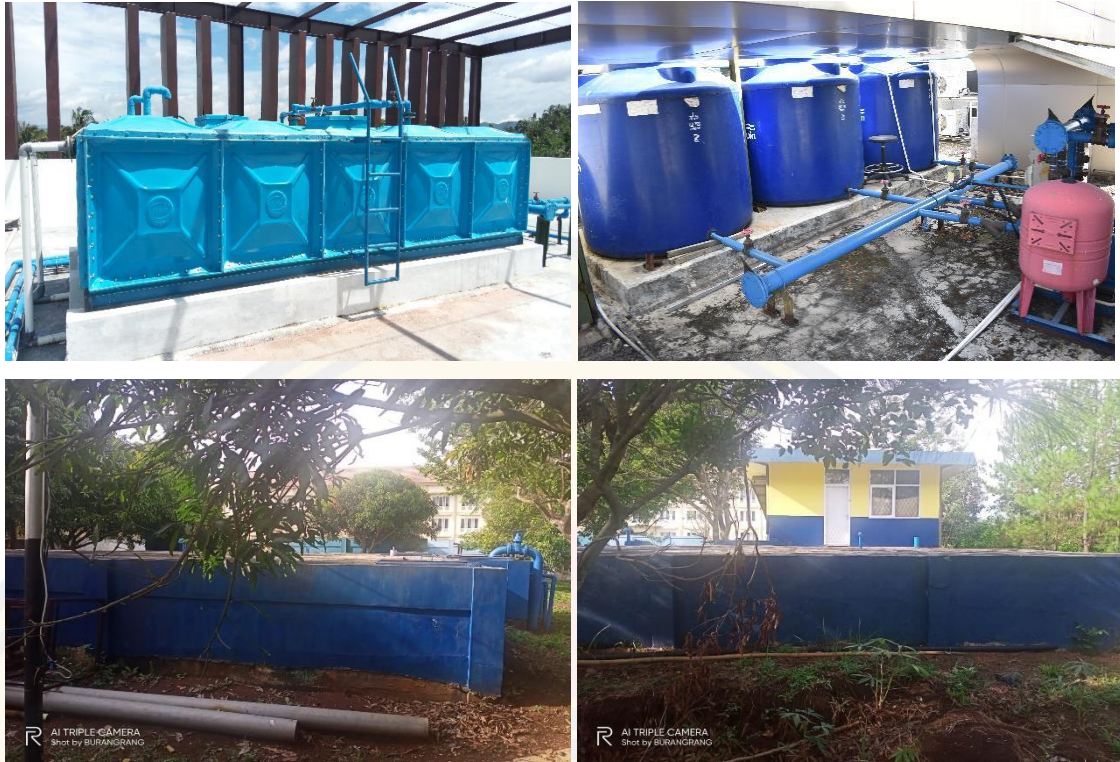
Figure 26. The Main Water Reservoirs at Universitas Padjadjaran
