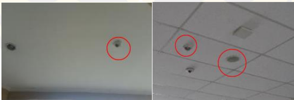
Figure 22. Integrated CCTV, Alarm, and Loudspeaker System
