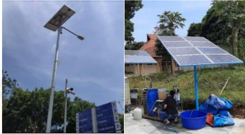
Figure 23. The Use of Solar Panels for Street Lighting and Water Pumps
