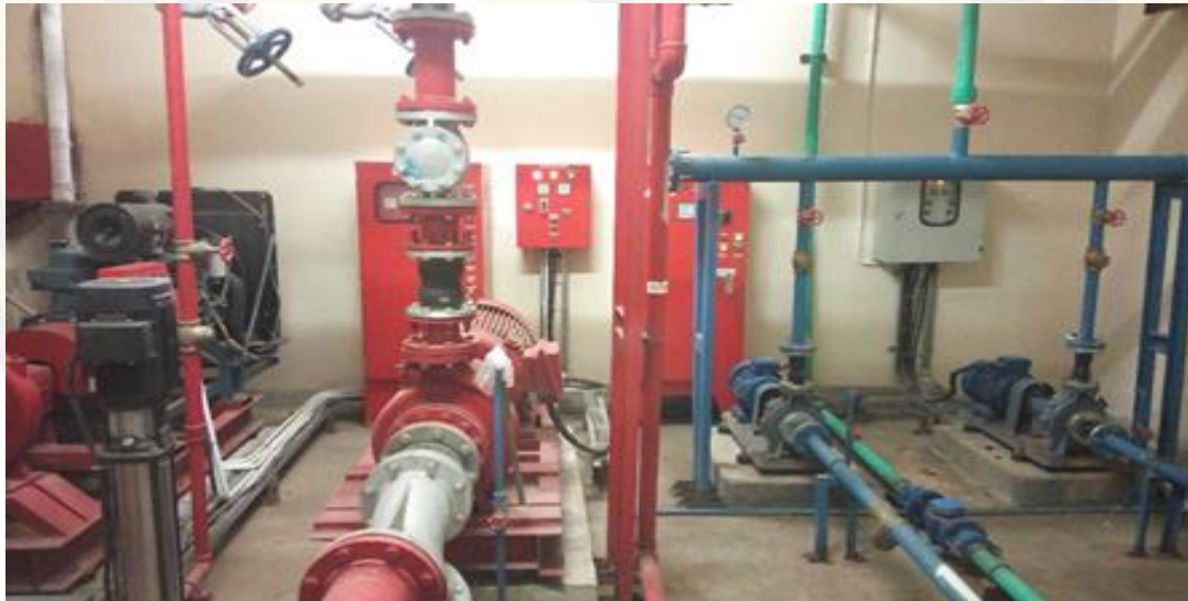
Figure 27. Well Water Installation at Universitas Padjadjaran
