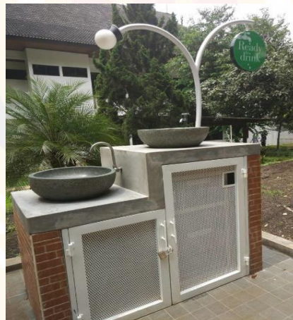
Jalatista drinking water recycling facility
