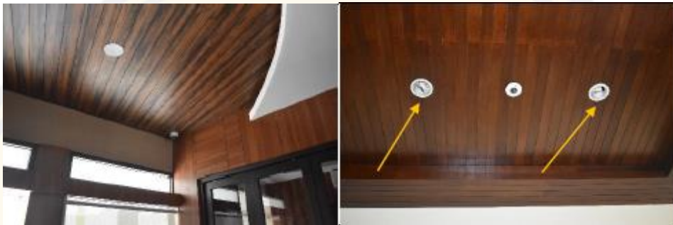
Figure 8. The Use of Energy-saving Lights
