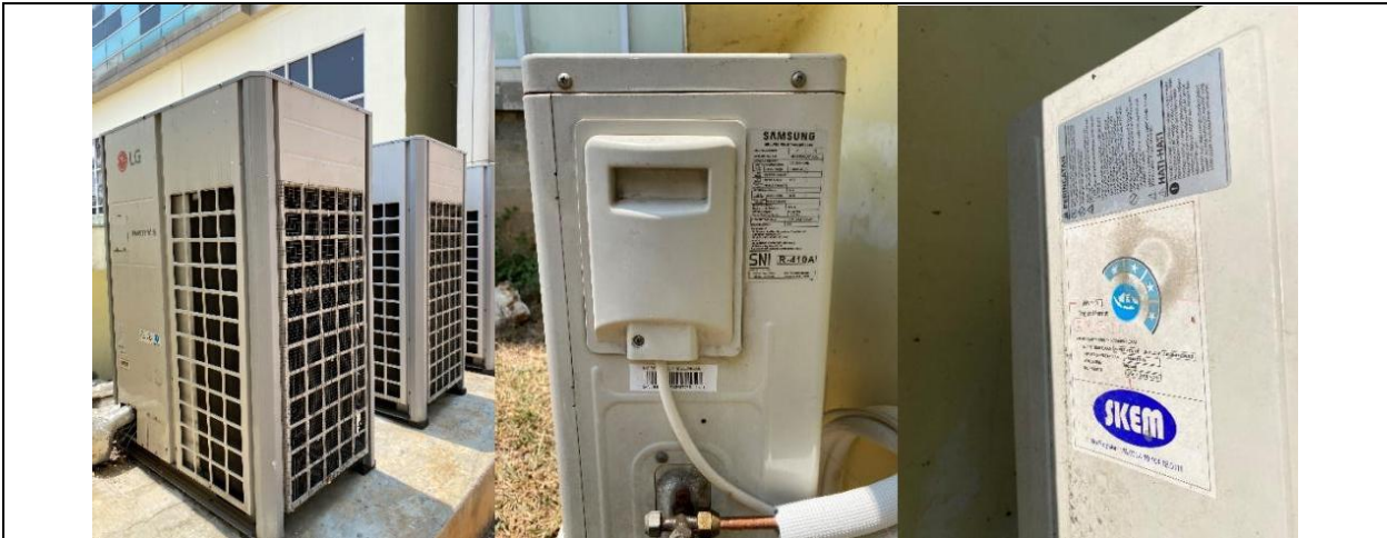
The use of ultimate efficiency air purification and ventilation (inverter AC).
